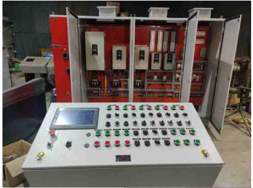
CONTROL PANEL WITH REMOTE DESK
