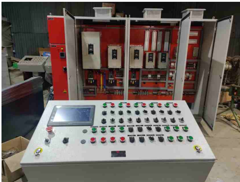
CONTROL PANEL WITH REMOTE DESK
