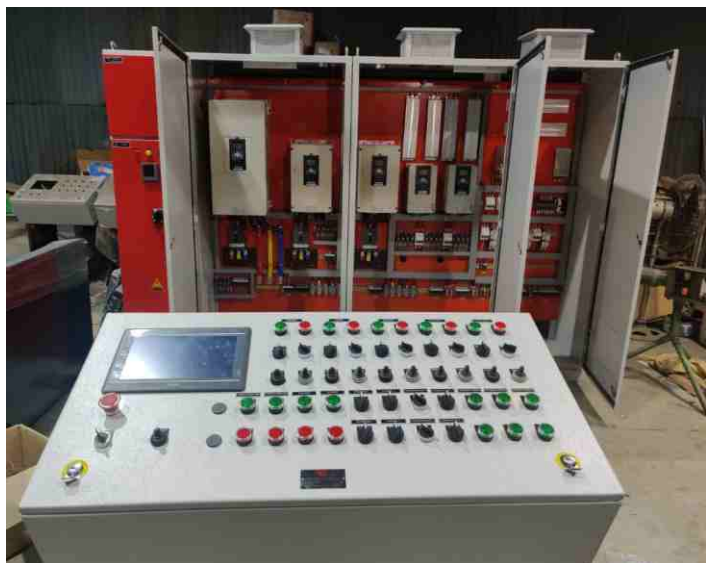
CONTROL PANEL WITH REMOTE DESK
